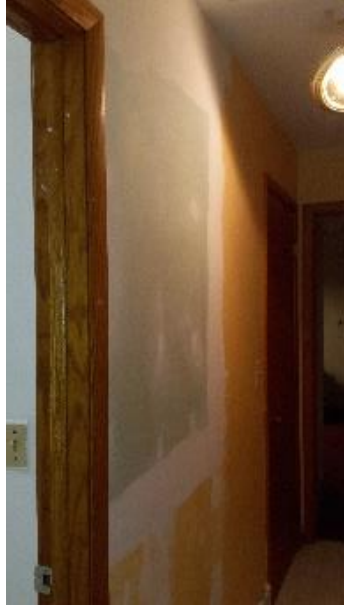
Finish Sanding and painting laundry room, bathroom and hallway on main floor
