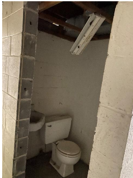
Remove toilet and sink. Cap of drain and pipes. Repair ceiling and light.
