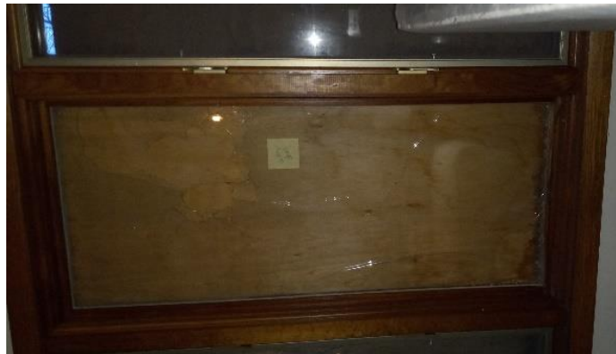
Replace broken windows and repair latches
